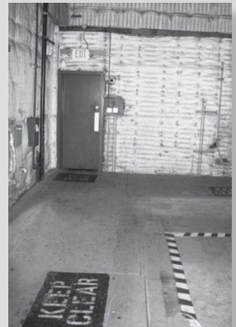
Figure 6.7. Fire lanes, whether on the buildings exterior (top) or interior (bottom), must be kept clear.
