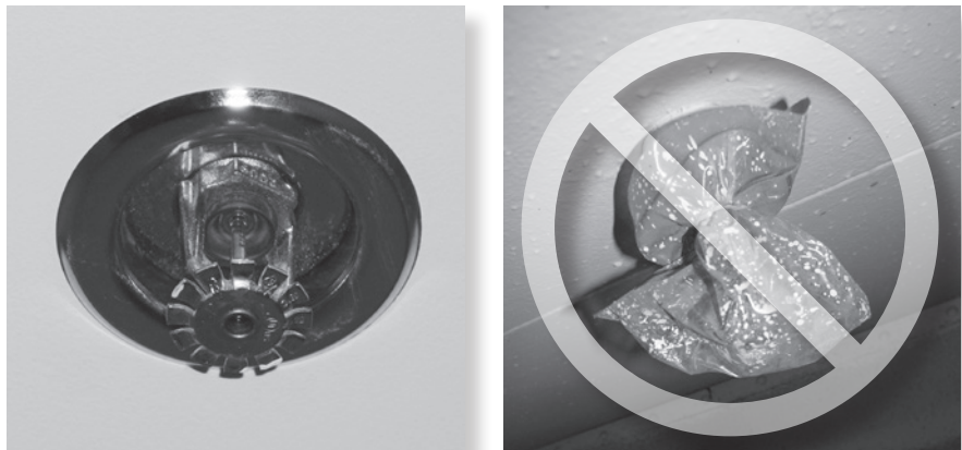
Figure 6.9. It is unsafe to cover sprinkler heads.
