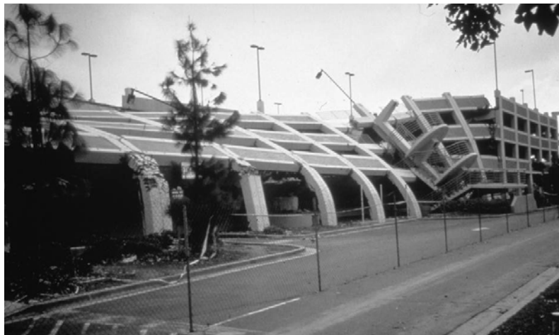
Figure 5.3. The magnitude 6.7 Northridge, California earthquake in 1994 illustrates the level of damage that could occur as a result of an earthquake, especially in urban areas. (Courtesy of NOAA, M. Celebi, U.S. Geological Survey.)
