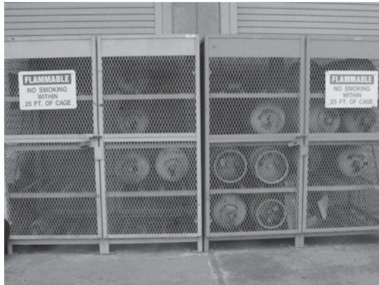
Figure 6.4. Outdoor storage for pressure vessels.
