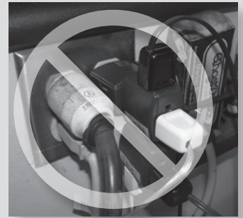
Figure 8.1. Plugging too many devices into one outlet can overload the circuit. When too many devices are connected to a small-gauge extension cord, excessive current overheats the wires.
