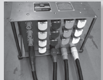
Figure 8.10. Examples of 480-volt systems.
