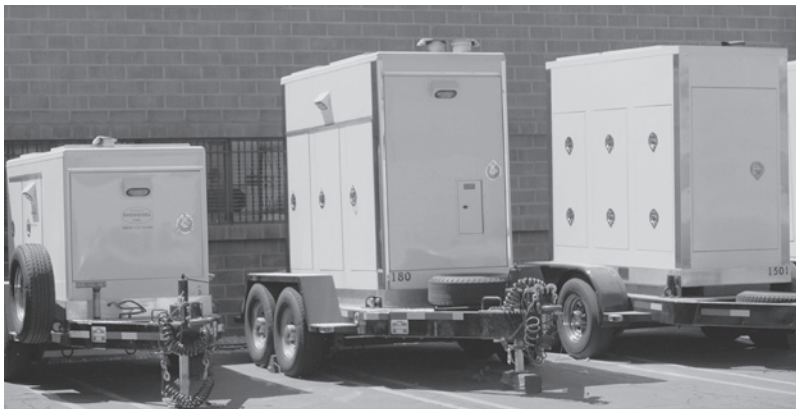
Figure 6.10. Fire extinguishers should be taken out of generators before use so that they are available if needed.
