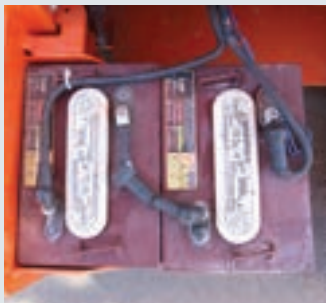
Figure 7.1. Rechargeable batteries in a scissor lift.
