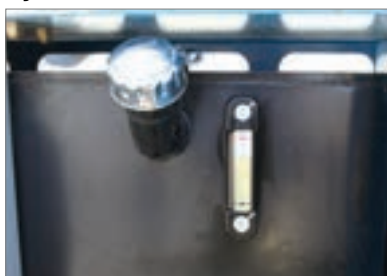
Hydraulic Fluid Tank
