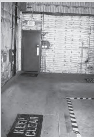
Figure 3.7. Fire lanes, whether on the buildings interior or exterior, must be kept clear.
