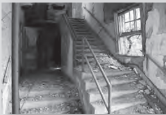
Figure 5.5. Flaking plaster and paint on older structures may release lead paint dust, which could pose a health hazard if inhaled or ingested.
