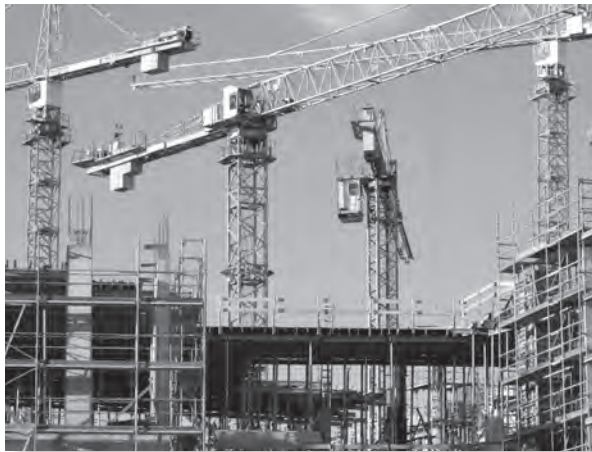
Figure 4.13. An active construction site may have unusual hazards such as moving equipment and high noise levels.
