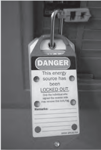
Figure 4.11. Lockout/tagout on an electrical switch ensures an employee working on circuits is protected from the risk of shock.
